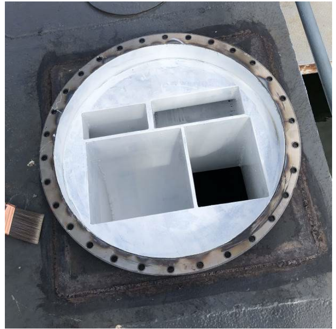
The custom-made manifold mounted to deck.
